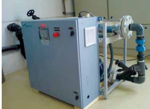
UV system at the Zuckerberg Water Institute.
