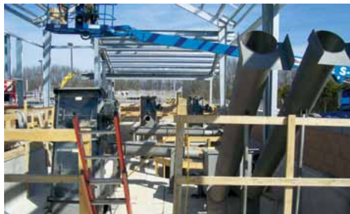
The plant's headworks under construction. At left: bar screen. At back: side-by-side band screens. At right: equipment washes and compacts screenings materials.
