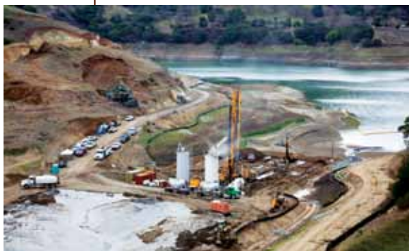
Contractor completes staging and begins work on grading the site for the construction of the new dam.
