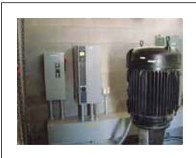
Employing variable-frequency drives gave the utility better energy efficiency and accuracy.
