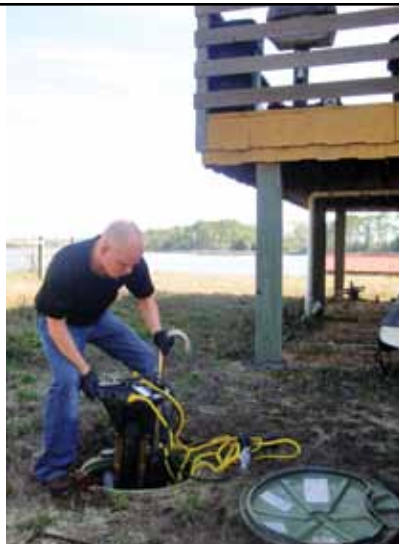
Carrabelle's pressure sewer system uses small-diameter pipes and grinder pumps installed at each home.
