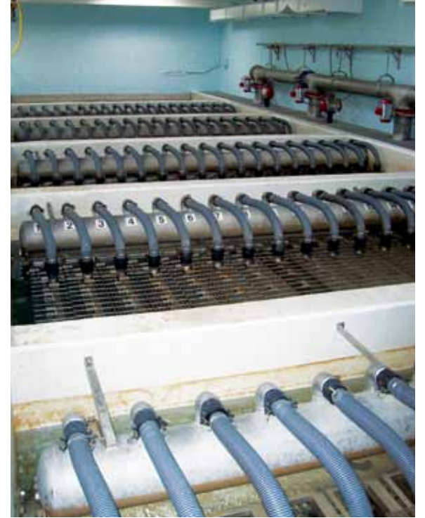
Manitowoc chose a new submerged membrane water plant that was retrofitted to an old sand filter plant.
