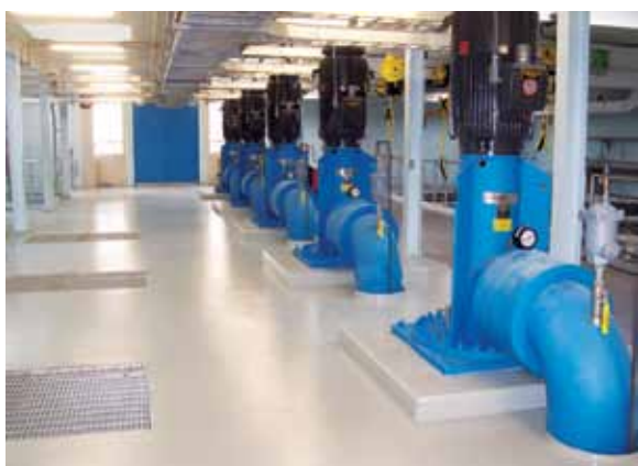
The team completed Manitowoc's new submerged membrane wastewater plant in 24 months.
