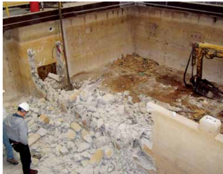
While Manitowoc’s new plant was retrofitted, several old concrete walls had to be demolished.
