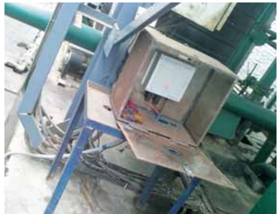
Physical methods to remove deposits can be maintenance-heavy and expensive.
