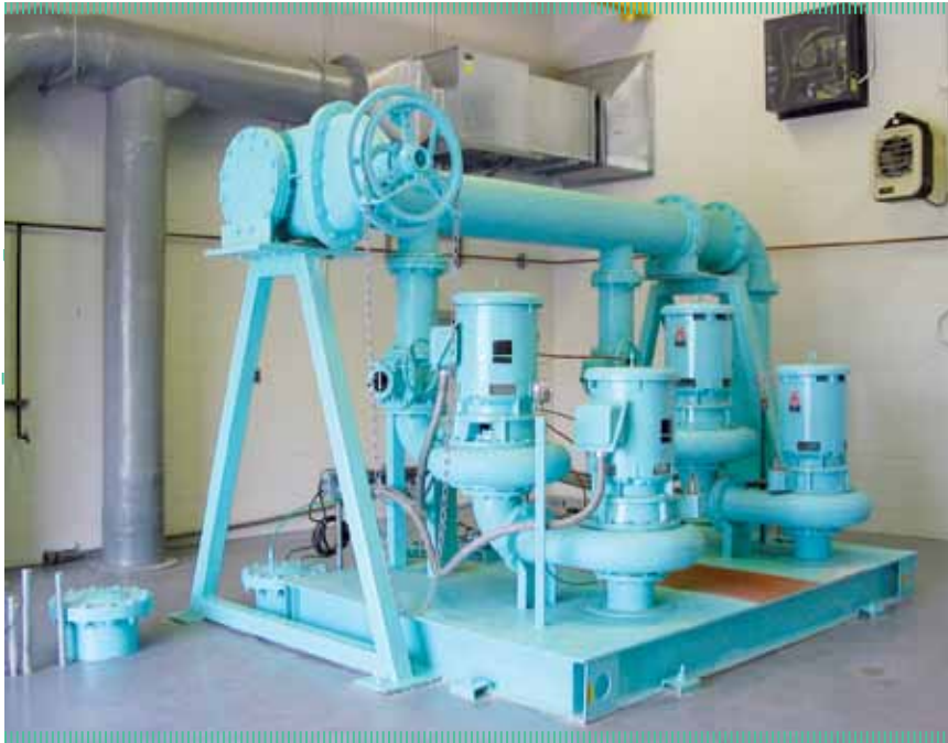
This vacuum-primed pump station serves a high-head pumping application in which a series pump arrangement operates at grade level with higher efficiency and less total connected horsepower.
