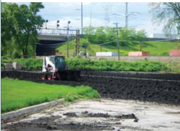
Biosolids are spread about 4 in. thick on an asphalt pad and bored over a three- to four-day period to dry.
