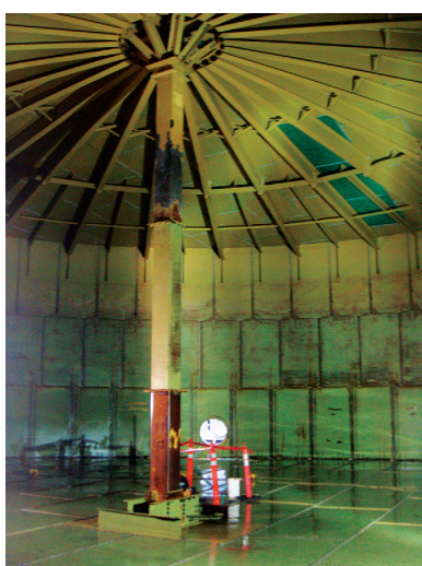
Interior of the Girdwood tank showing damage to the center column
