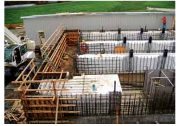
One truckload of EPS geofoam contains the equivalent of 12 dump trucks of earthen fill.
