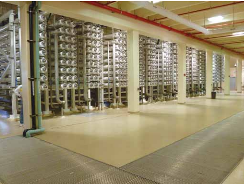
End view of Jupiter, Fla., plant's five nanofiltration trains
