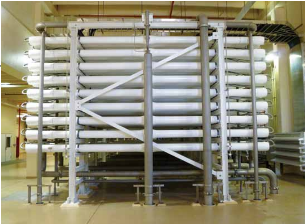
Side view of a Jupiter nanofiltration train depicting the vessel center exits and collection piping
