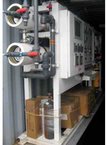
RO membrane units and instrument panel at Laguna Madre Water District Seawater Desalination Pilot Plant
