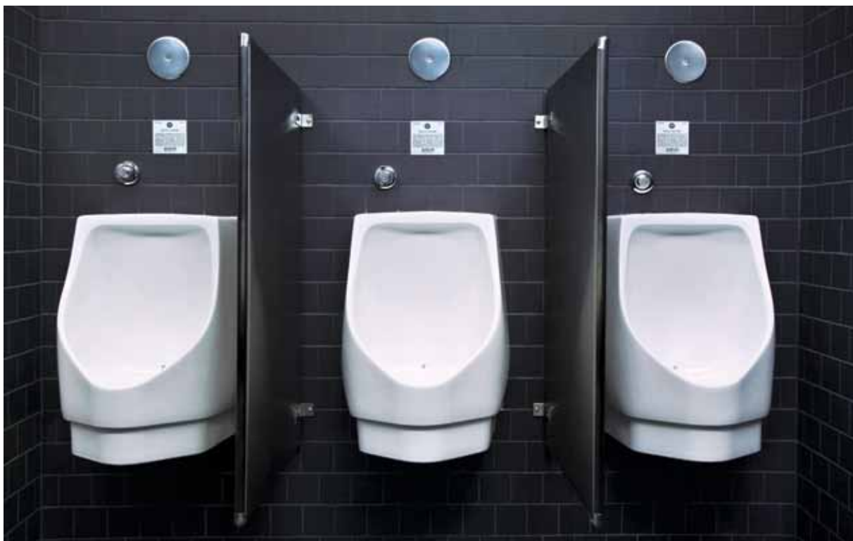
Waterless urinals at Disney Concert Hall in Los Angeles
