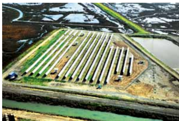
Oro Loma Sanitary District pursued solar panel installation after an energy audit inspired facility managers to reduce high operating energy costs.
