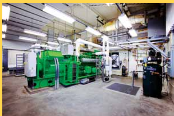
1.7-MW cogeneration facility
