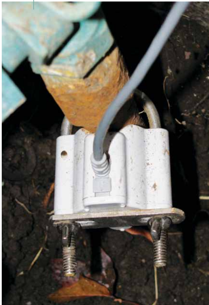
A leak detection sensor on a water pipe
