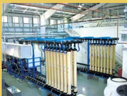
Water undergoes a tertiary treatment process before it is discharged into the lake.
