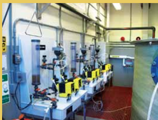
Chemical pump skids
