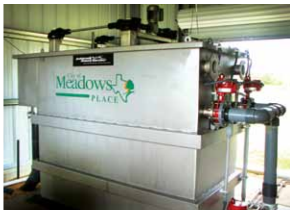
The filter and collection system provides at least 200,000 gal of Type 1 reclaimed water per day.
