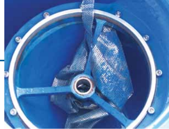
Debris lodged in the lower guide and seat area of the ACV
