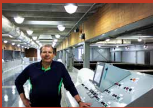
Pete Muncaster, Marston WTP supervisor, said that the plant's partnership with the U.S. Forest Service will improve water quality and add capacity.
