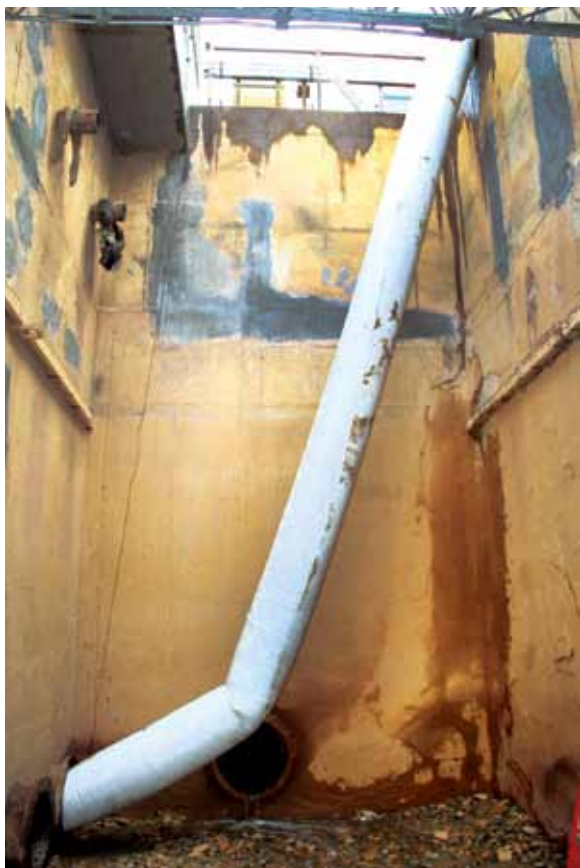
Top: The six water effluent lines in need of repair ran beneath the plant's treatment tanks. Bottom: The installation crew applied extra pressure to help the resin-saturated liner navigate the bends in the lines.
