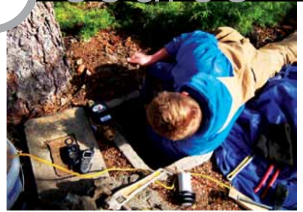
As part of the AMR upgrade in Coeur d'Alene, Idaho, Kyle Marine, crew utility supervisor, replaces one of the utility's 17,500 meter endpoints with a new meter and absolute digital encoder register.
