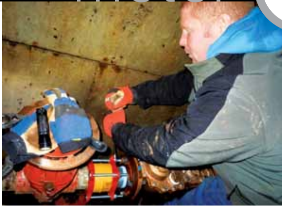
Utility worker Josh Mayne installs a new 3-in. meter at a commercial site.
