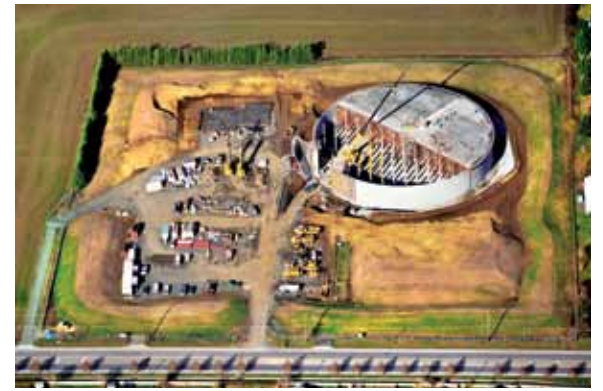
The tank and pump station under construction in February 2013. Photo courtesy of Brad Phelps, CH2M Hill
