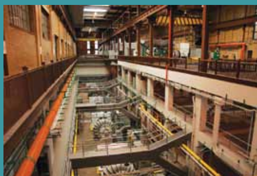
A view of the pumps and blowers
