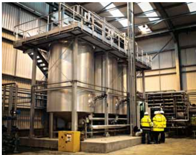
A three-tank batch pasteurizer system for the treatment of mixed food waste
