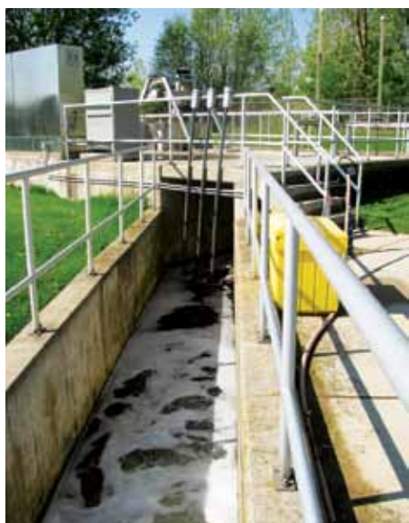
The effluent channel of the Adelaide facility with the effluent probes measuring DO, pH, temperature and TSS
