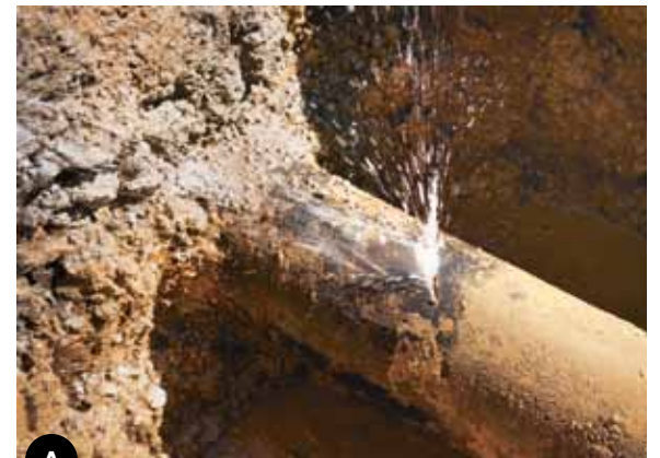
A Snapshots of cut pipe from an excavation in Sausalito, Calif.
