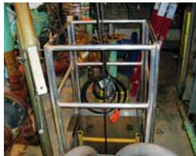
The entrance to the sump where an employee must work beside a 600-V submersible pump
