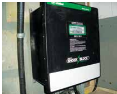
The answer to pump shock protection was to install an equipment ground-fault protection device.
