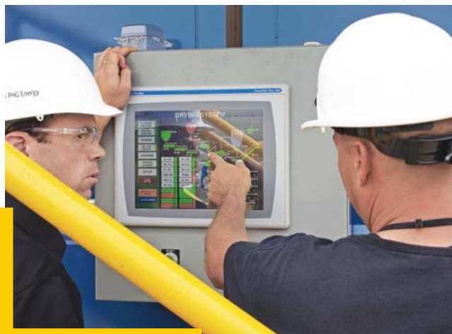
HMI control and monitoring systems at the plant
