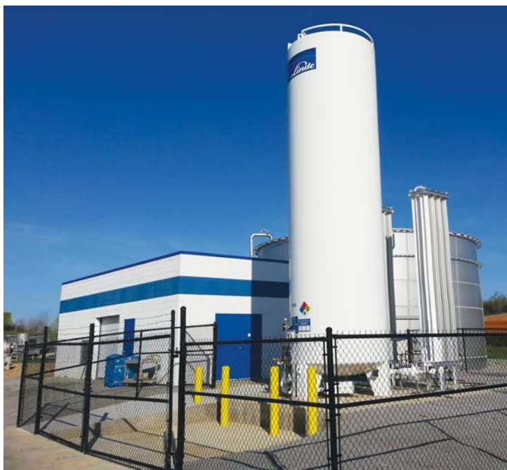
The plant's 6,000-gal liquid oxygen tank
