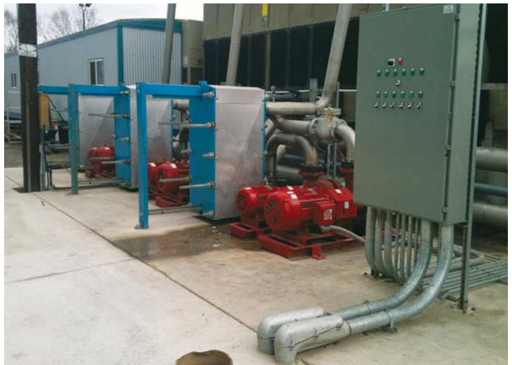
The plate and frame heat exchangers seen here are an ideal fit for smaller plastic cooling tower models, which complement the compact footprint that is important to many industrial process applications.
