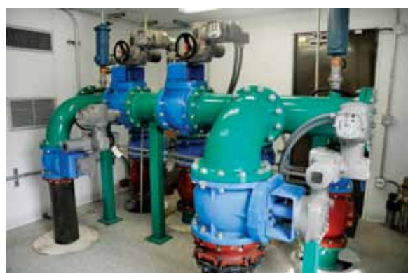
The station houses two separate force mains, automatic valves and four pumps.
