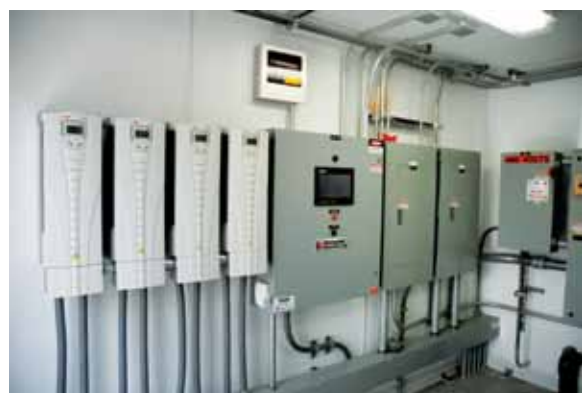
The upgraded control panels were custom designed and built into the original SCADA system.
