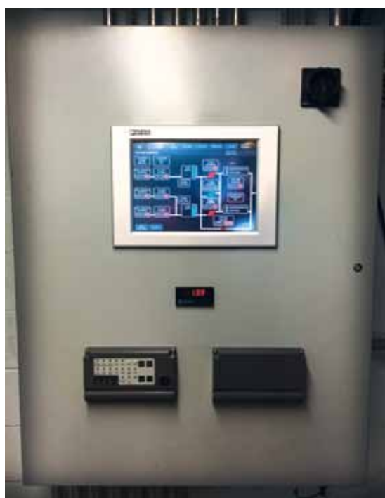
New control systems allow for wireless communication and remote monitoring.
