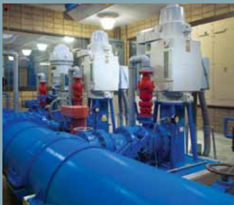
Top: The treatment plant is owned by Ottawa County and operated by the city of Grand Haven. Bottom: High-service pumps
