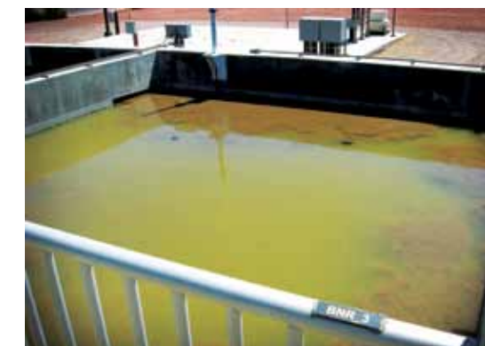
BNR anaerobic cell No. 2 without mixing
