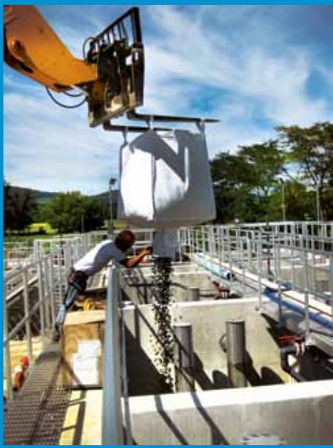
The carrier media provide high specific surface area for biofilm growth, allowing the plant to handle increased daily flows.
