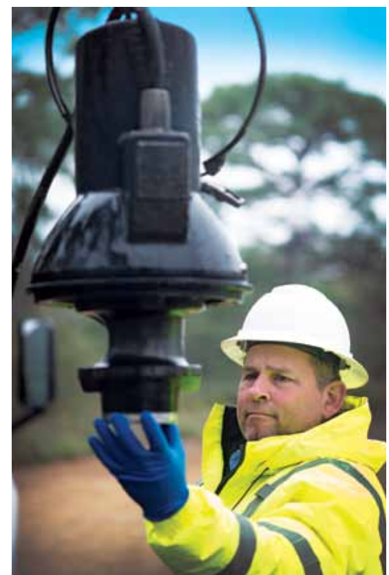
Less grease buildup in the wetwells has led to reduced maintenance costs for both entities.
