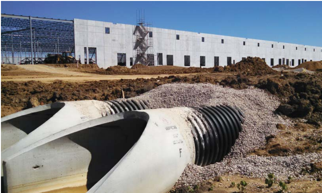
HDPE pipe connects to concrete aprons to provide an outlet for the system.
