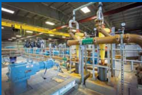
The Rueter-Hess Water Purification Facility employs one of the few recirculating powder-activated carbon systems in the U.S.
