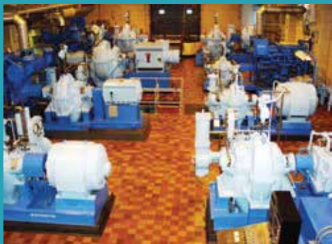
The Evanston Water Treatment Plant's nine high lift pumps have a total capacity of 147 mgd.
