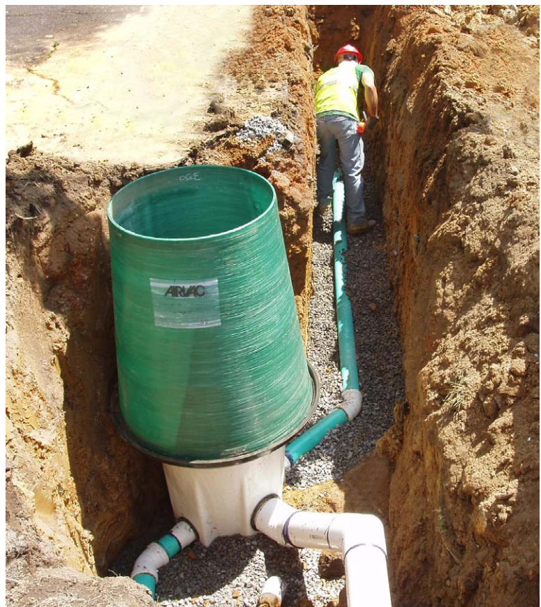
Gravity lines transport wastewater from the home into a buried valve pit.
