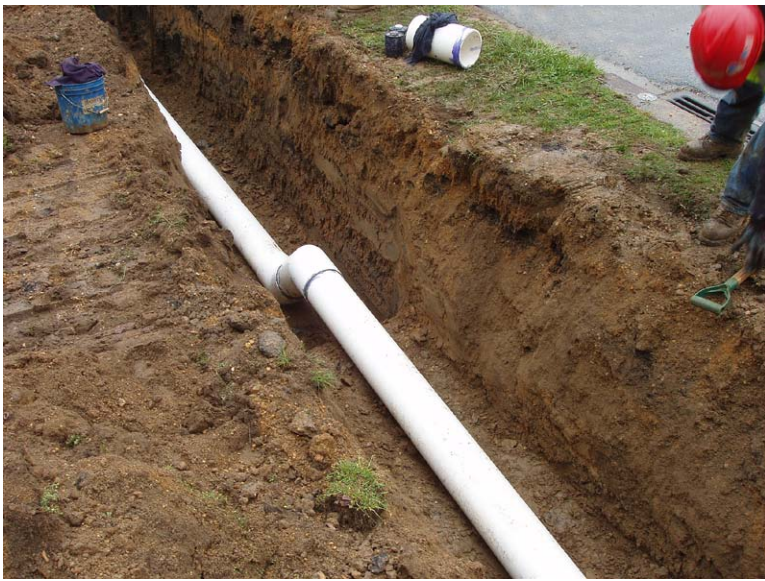
Vacuum mains are laid in a sawtooth fashion to insure adequate vacuum levels at the end of each line.
