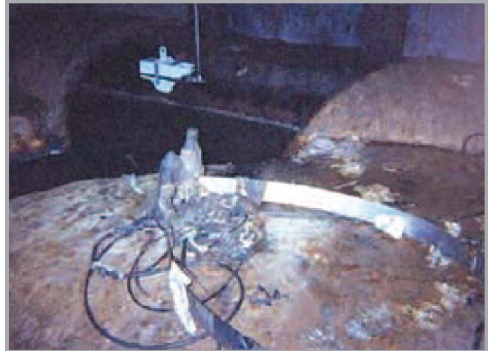
Figure 6. Fouled Submerged Type Sensor
