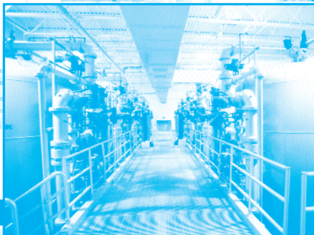
12,000 GPM Countercurrent Regenerated system operating in Illinois
