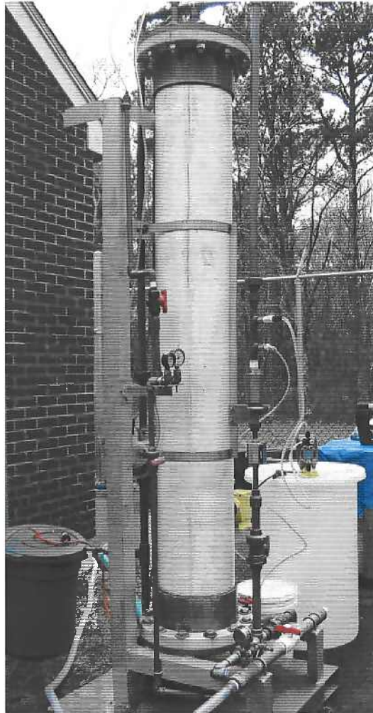
FIGURE 3-4 LAYNEOX PILOT VESSEL
