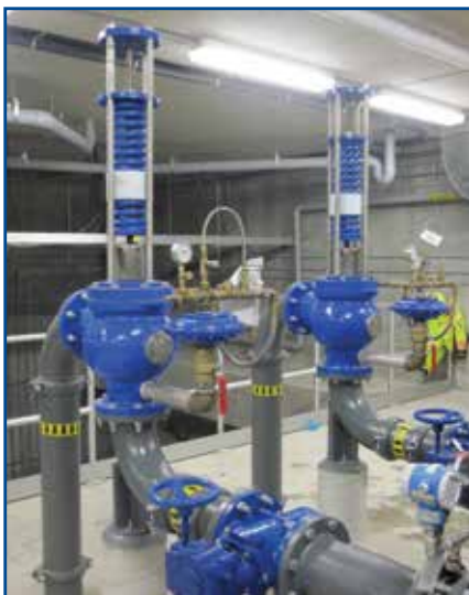
Region of Peel installation - Ontario, Canada
