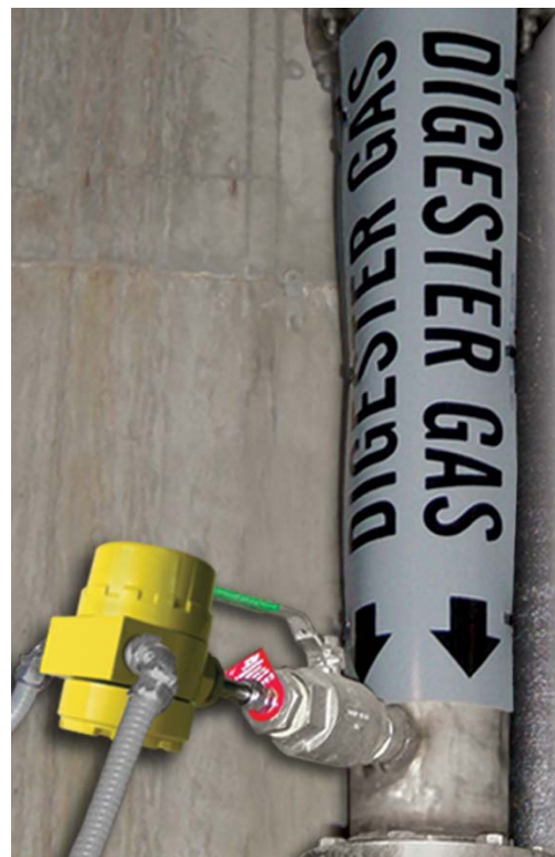
Figure 5: Flow meter installed on digester gas pipeline
