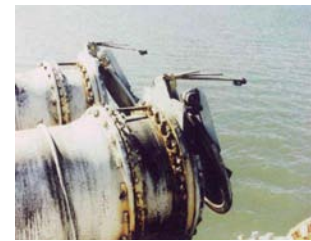
Figure 3 - Failed Open Swing Flap Gate
