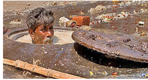
Figure 2 - Man Unclogging Sewer Overflow in Chennai, India
