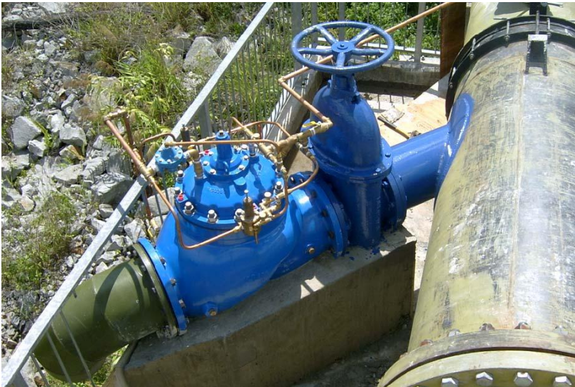
Figure 17: Malaysian surge anticipating relief valve installation
