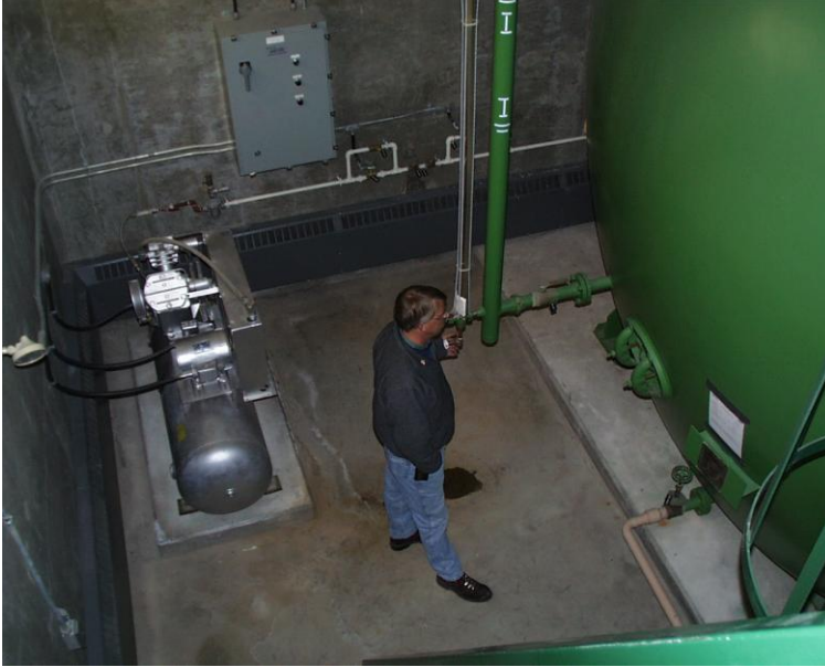
Figure 13: An example of an installed surge tank located indoors
