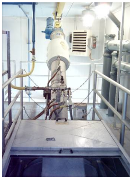
Figure 35 – Rotary Drum Screen RPPS with 3mm hole openings
