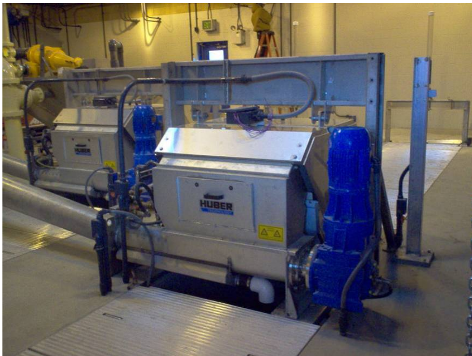
Figure 37 – Screenings washer/compactor behind a step screen in Reno Stead, NV
