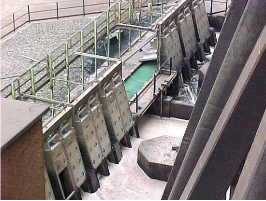
Figure 14 – SSV for cooling water intake
