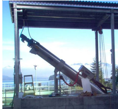
Figure 4- Ro2 installation in Alaska (with frost protection package)
