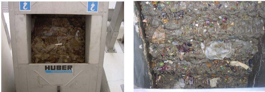
Figure 12, 13 – Proper screenings mat for a Step Screen
