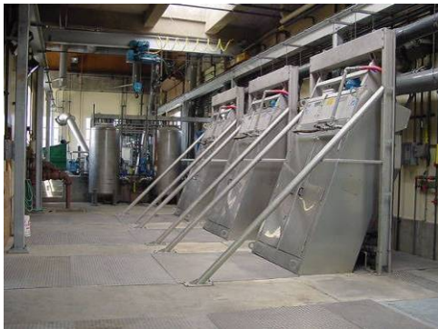
Figure 10 - SSV + Vacuum Conveyance System at North Davis, UT
