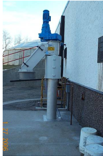
Figure 31 – RoK4 outdoor installation in Elroy, Wisconsin
