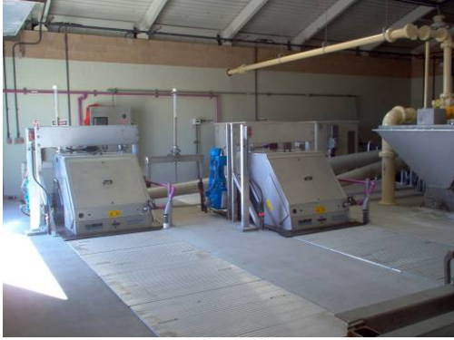
Figure 6- Step Screen at Reno Stead, NV
