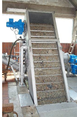
Figure 21 – Perforated band screen (covers removed)
